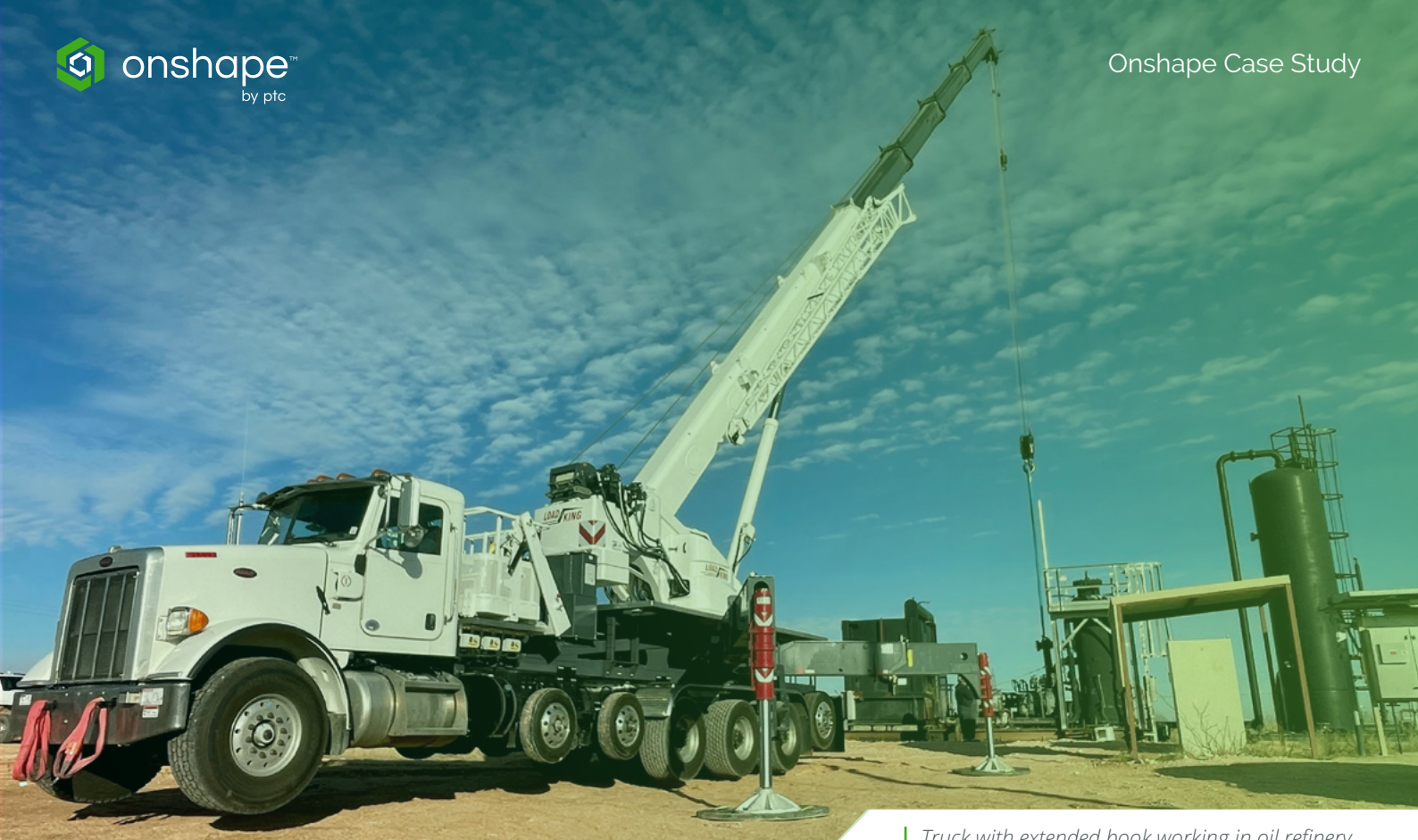
| Truck with extended boom working in oil refinery
